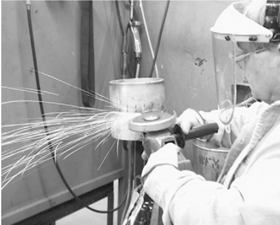
Figure 304-3.1-3 Grinding of Weld Flaw
